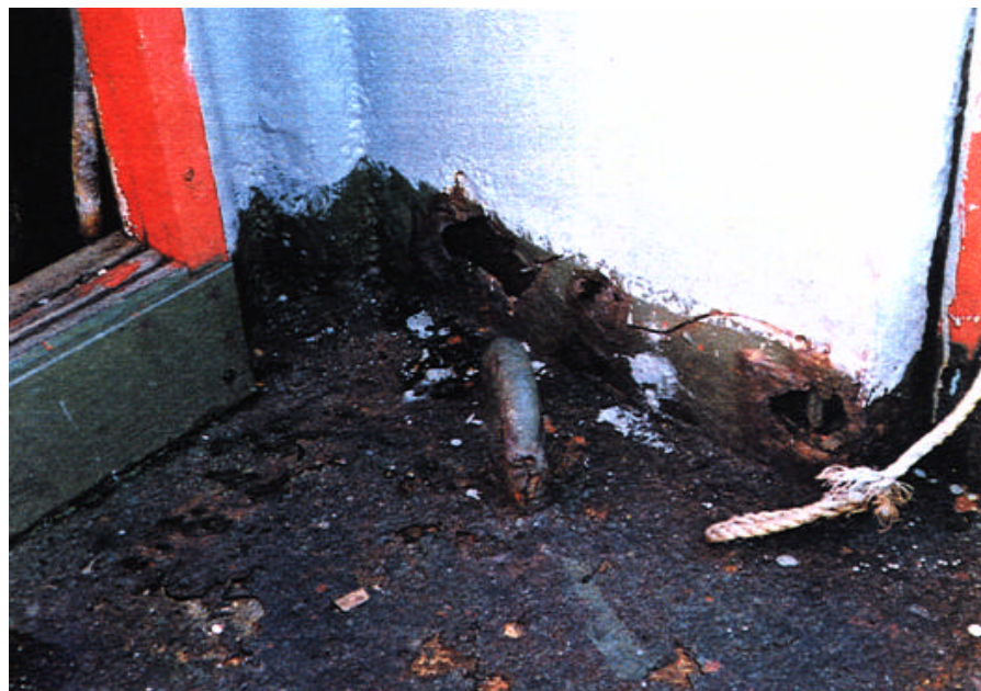
Photograph 1 Corroded accommodation house side structure
